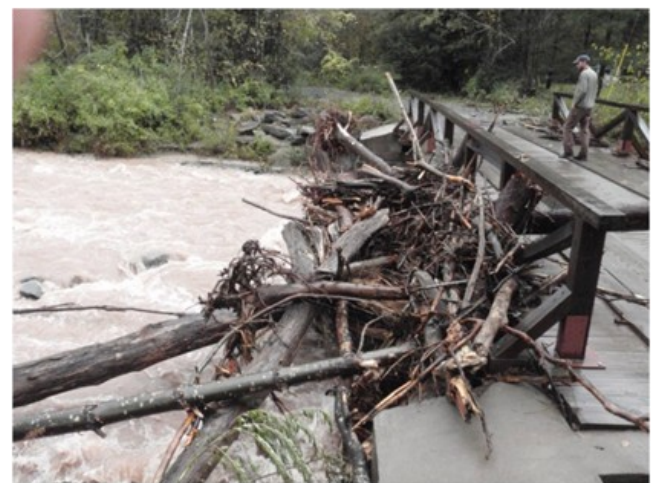
Woody Debris can cause damage to bridges if not removed or there is not enough space for the debris to pass under the bridge
