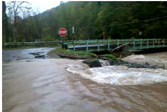
Brown Road in Olivera, damaged by flood water by McKinley Hollow Bridge
