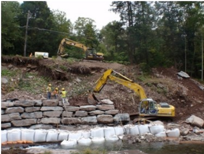
Rock is placed at the toe of the eroding slope on Woodland Creek. Large sand bags prevent construction runoff into the stream
