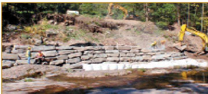
Above: AWSMP staff coordinated the design and installation of road protection projects.
